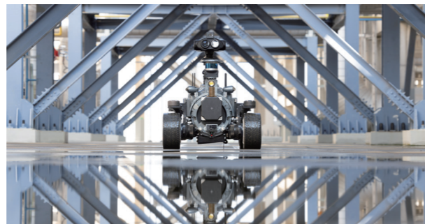
Intelligent inspection robots conducting frequent patrols across the site
